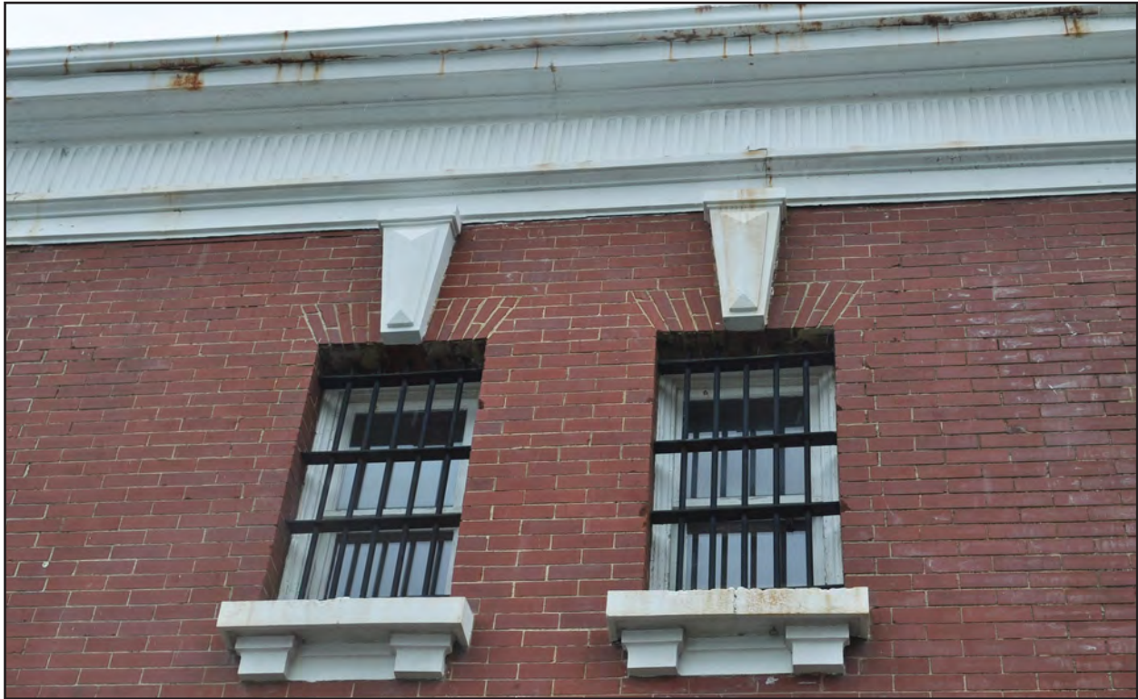
Figure 79. Rockingham County Jail, Rockingham County Jail, Concrete Cornice and Window Detail, West Side
